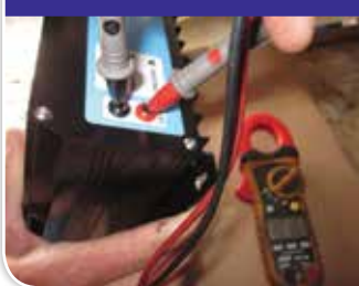
DC Voltage from PV Panels
